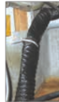
Crushed vent ducting, will impede proper and safe venting of fumes. Replace damaged duct
